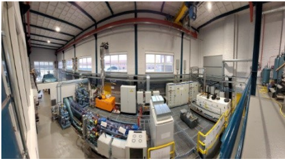
The physical Zero Emission Lab, containing a fuel cell, hydrogen, a modern dual fuel generator set, and sophisticated electrical power distribution.
