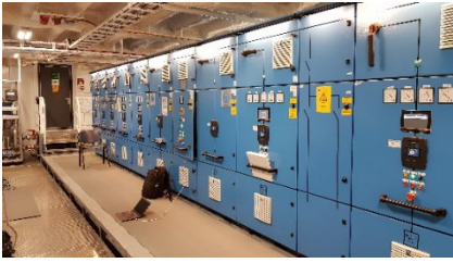
Power measurements on board.
